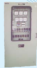
Solar Charge controller
